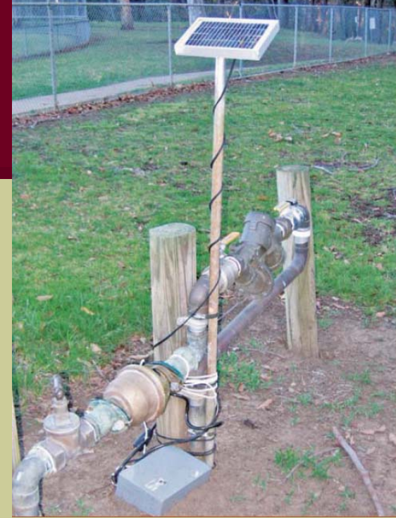
Solar-powered smart water meter Source: Hauber-Davidson and Idris (2006)
