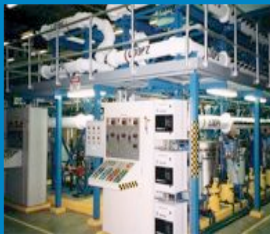
Simulated drinking water distribution system
